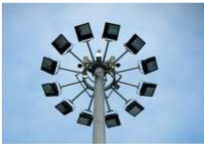
Solar Street Light- High Mast
