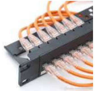
Passive Network - Cat6/ Patch Panel
